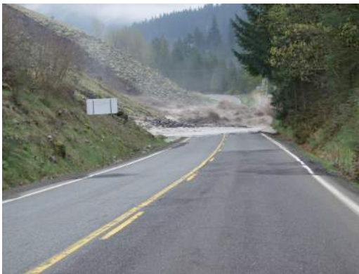
Canal Water Escaping Embankment Breach onto Local Highway
