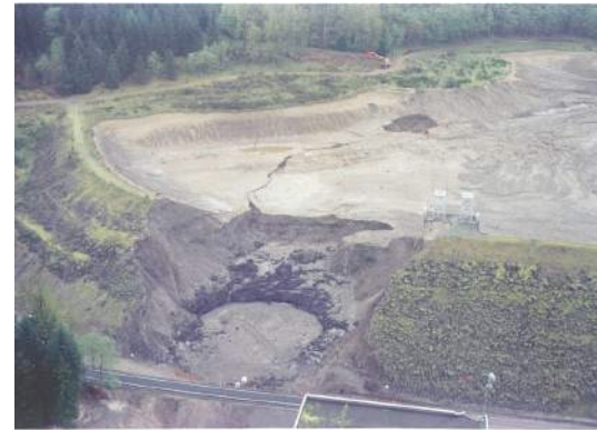
Blowout Failure Under Canal Embankment-Empty Canal
